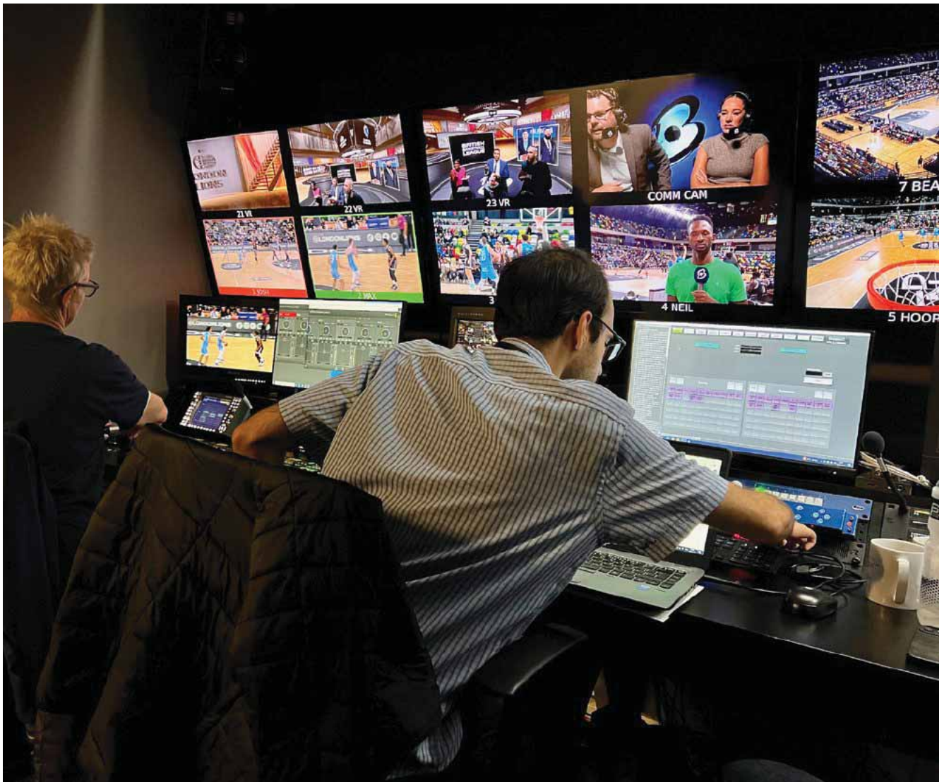
Remote racking at EBC of Studio and OB cameras.
